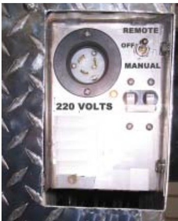
Fig. 4. Turn Off Main breaker at blower and at main panel when not in use.
