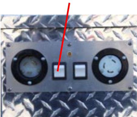
Figure 1. Turn Off Main breaker at blower and at main panel when not in use.
