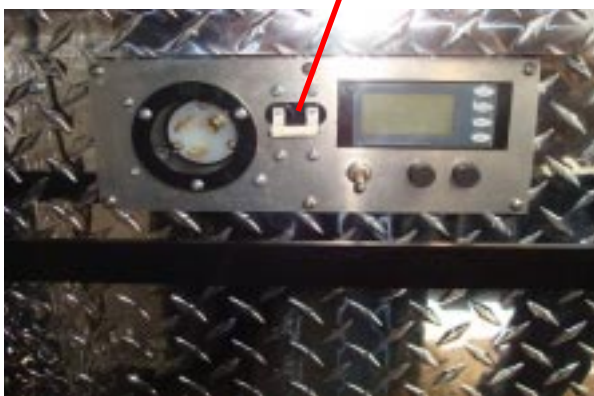
Figure 1. Turn Off Main breaker at blower and at main panel when not in use.
