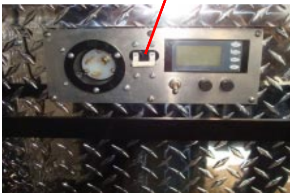
Figure 1. Turn Off Main breaker at blower and at main panel when not in use.
