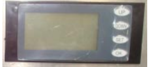
Photo 8 Combination power & hour meter
